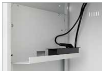
Power distribution unit shelf
